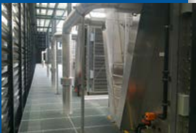
▲ Amsterdam University also benefits from the new concept as a neighbour of the data centre, which provides it with surplus heat for its heating.
