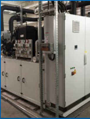
▲ The chiller's compressors are provided with an acoustic canopy.
