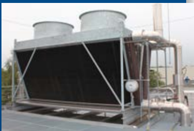
▲ The unit is equipped with glycol collection basins.
