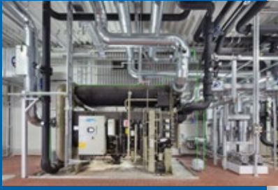
▲ The two central absorption chillers are enclosed for sound insulation purposes.
