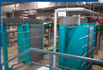
▲ ...more than 25 MW must be provided
