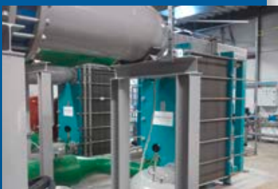
▲ thermowave plate heat exchangers in operation...
